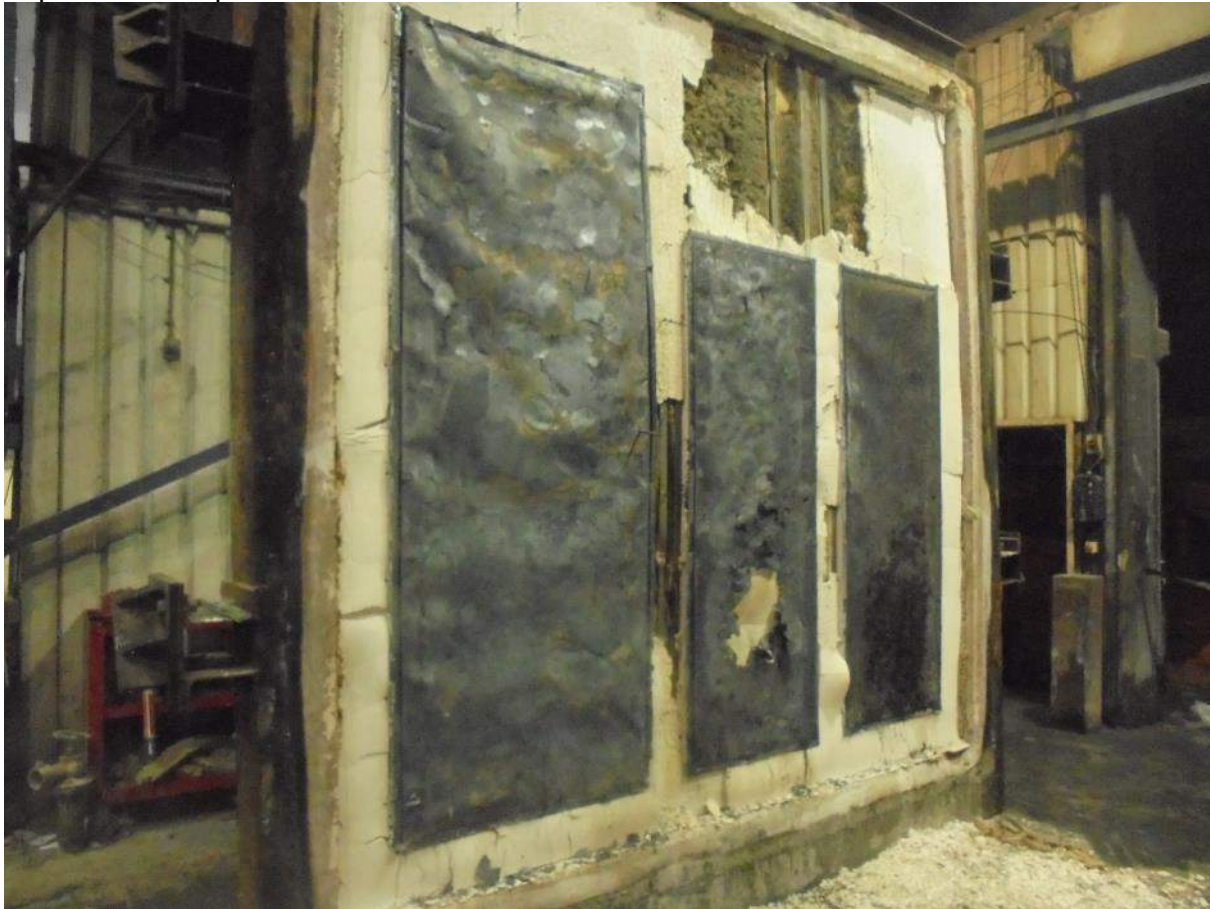
Exposed face – post test
